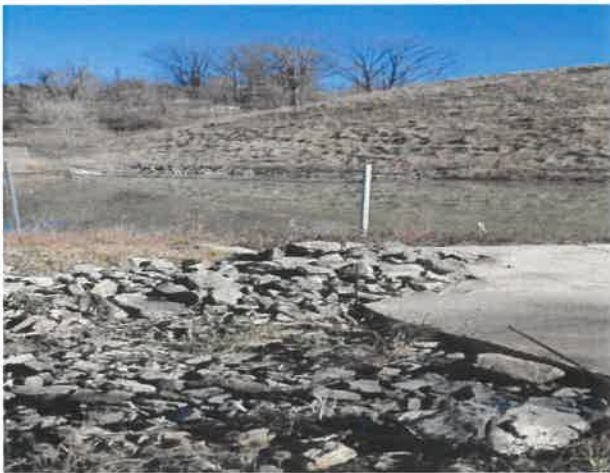
Storm water pond and drainage
